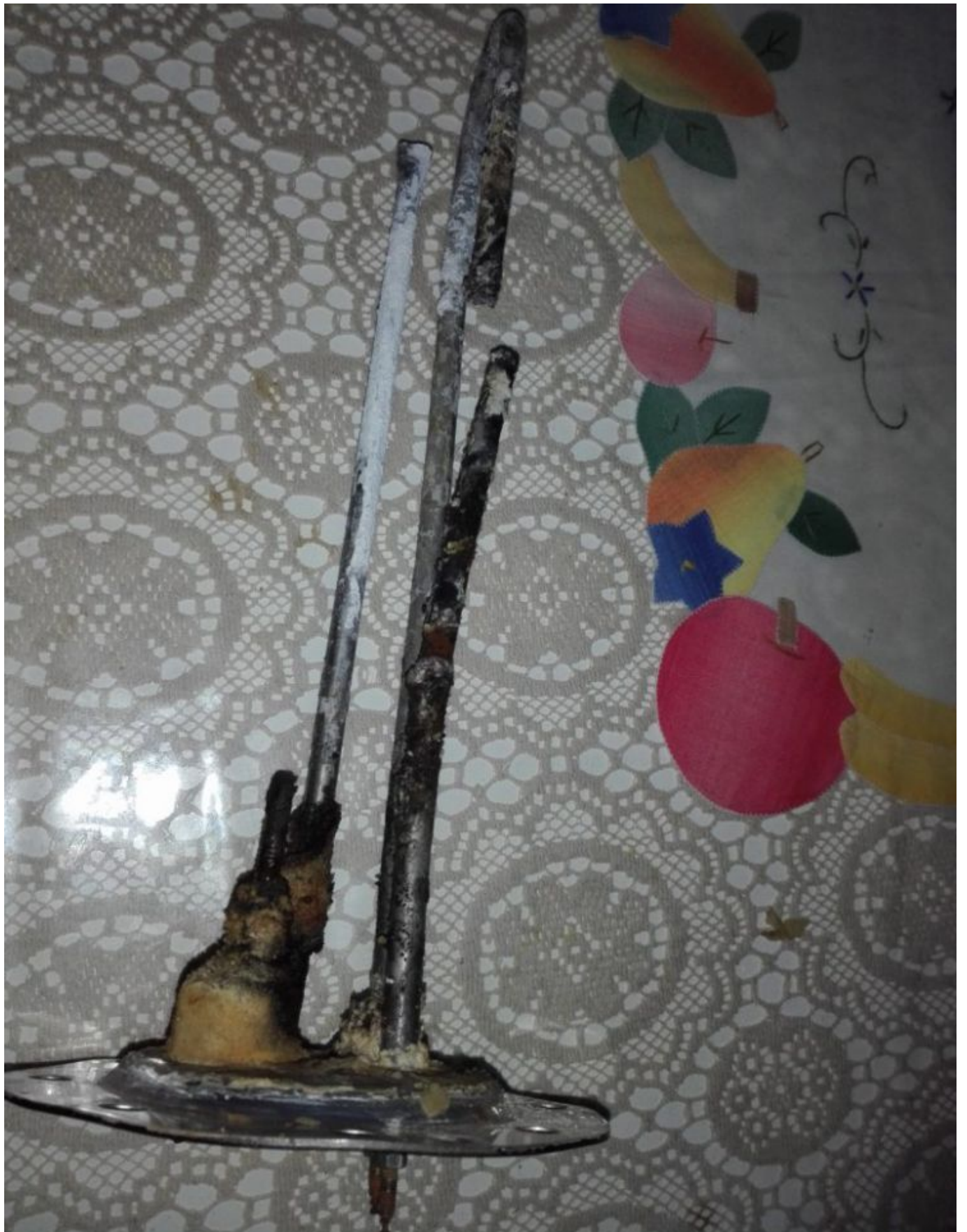
Solar water heater maintenance error
