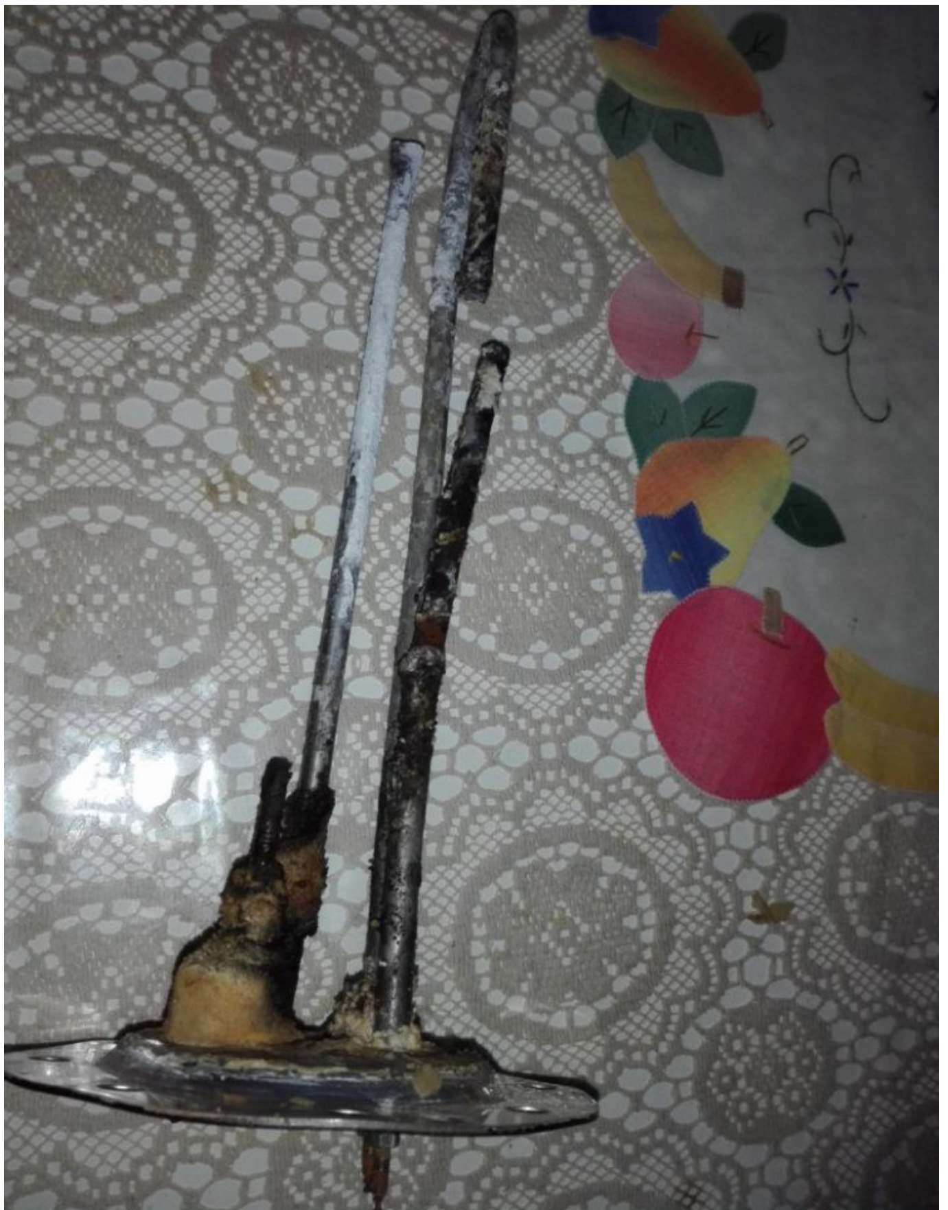
Solar water heater maintenance error
