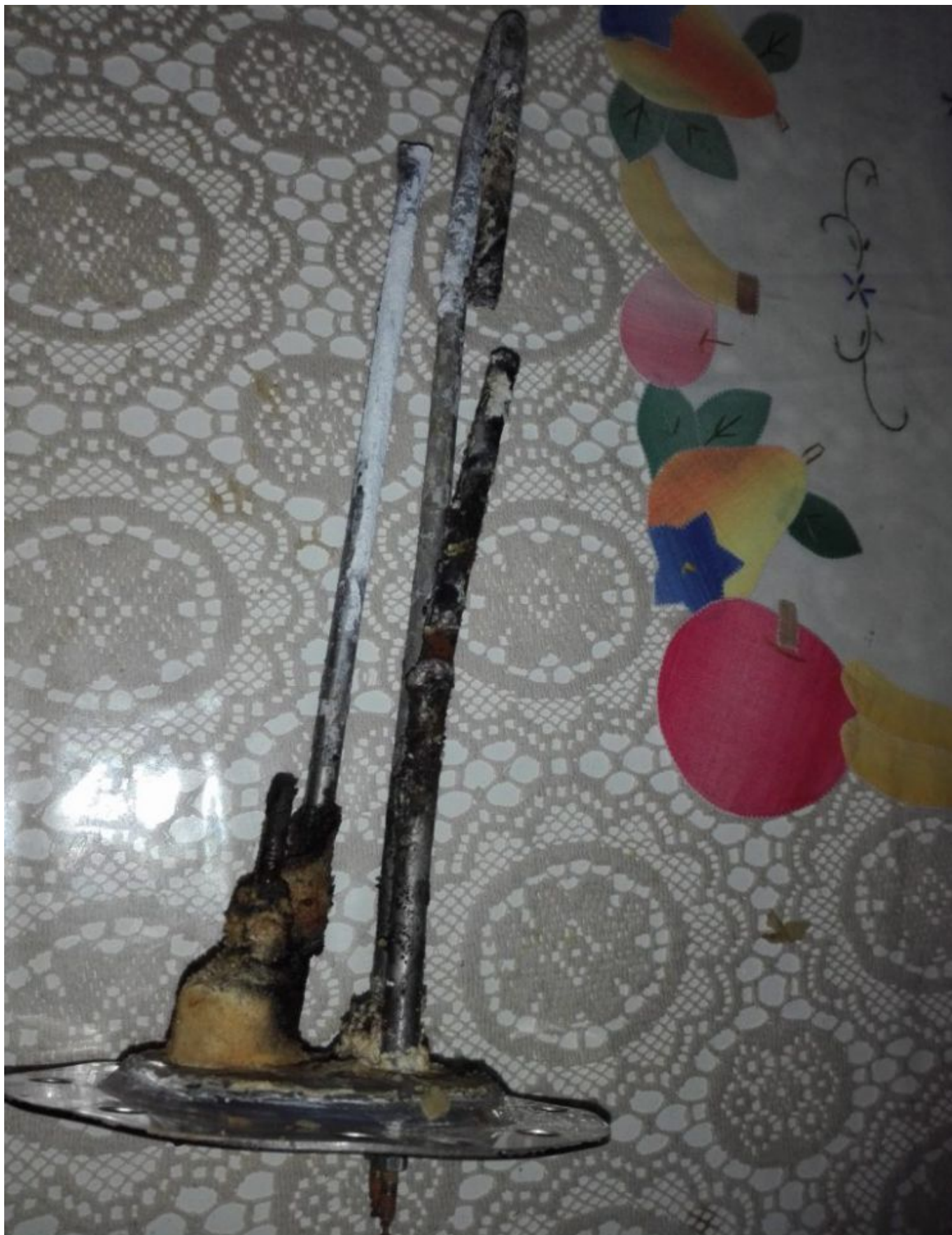
Solar water heater maintenance error
