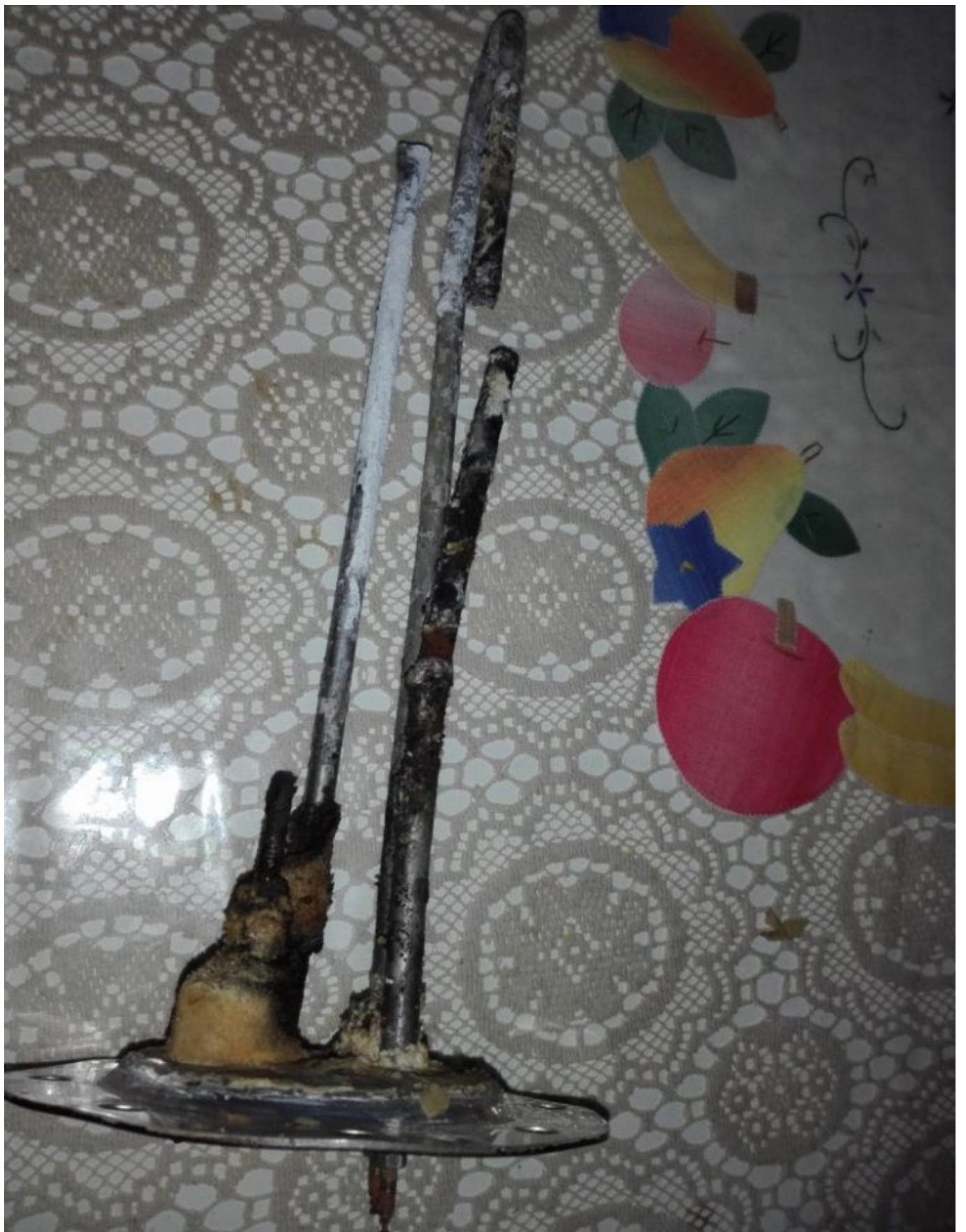
Solar water heater maintenance error
